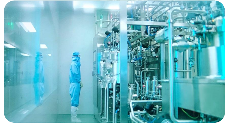
Dedicated production equipment installed in our factory
